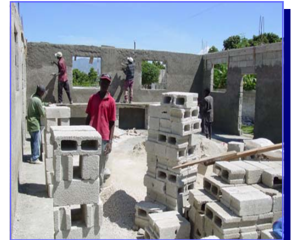
CONSTRUCTION CONTINUES ON THE FIRST SEVENTH DAY BAPTIST CHURCH IN CROIX DES BOUQUETS, HAITI
